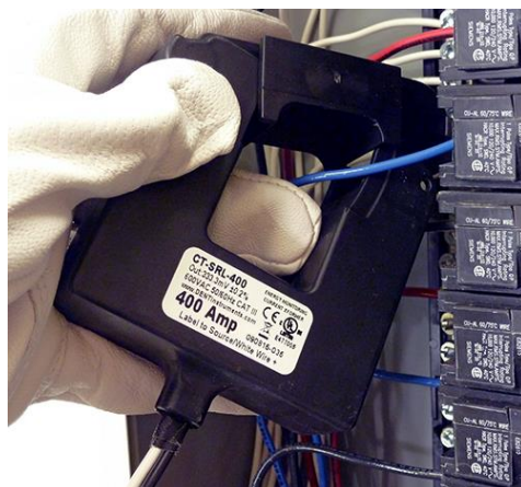
Photo 2: Install CT Around Conductor.
